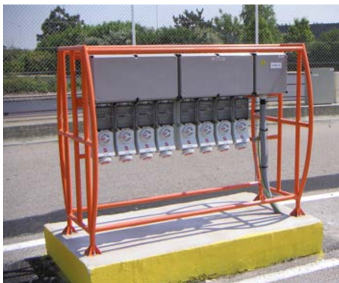
Container Terminal, Le Havre – France
